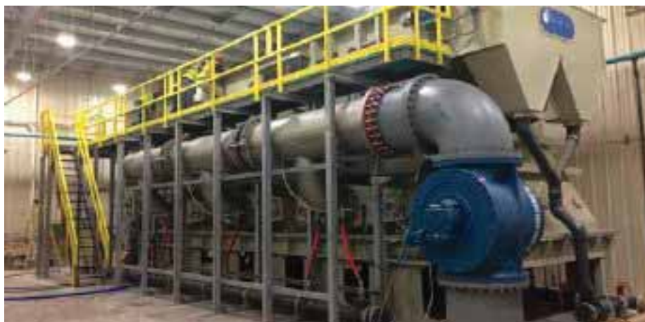
The Ideal Dissolved Air Flotation system installed at the Hopewell Regional Wastewater Treatment Facility. Photo credit: World Water Works
